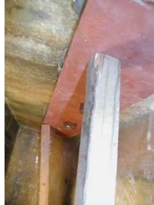
ARG installation surface (bottom view)
