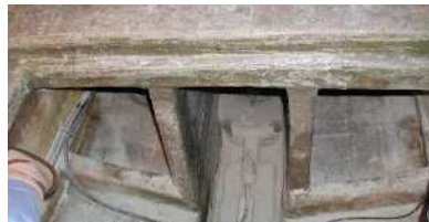
ARG installation surface (side view)
