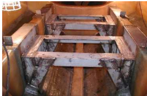
Example of setting up iron trestle for FRP ship Figure 3-2 Reinforcement of ship
